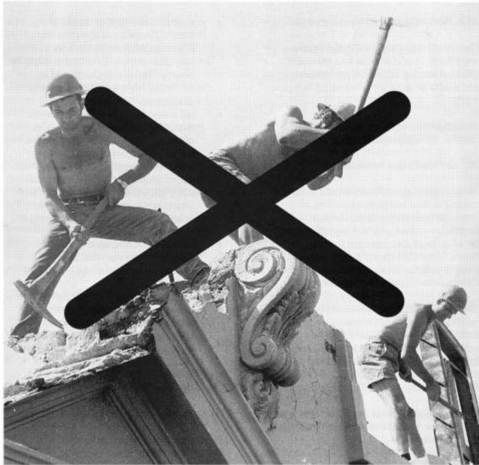
Figure 13: Example of unsafe demolition work. Safe working platforms have not been provided and the clothing used gives too much exposure to the sun
