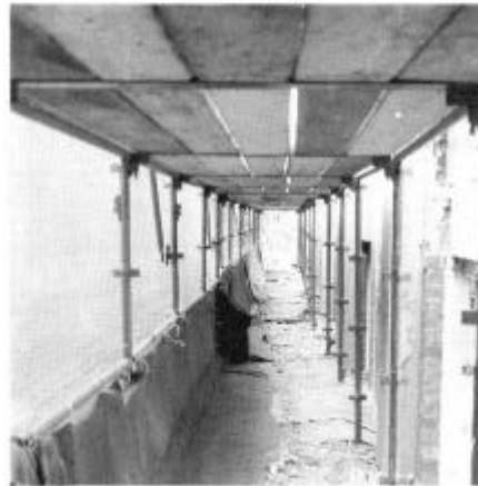
Figure 12: Perimeter scaffolding sheathed with old carpet to prevent debris from falling. The carpet is thrown back inside the building when demolition on that level is finished
