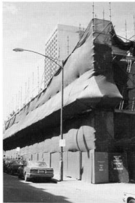
Figure 11: Perimeter scaffold on a narrow pavement. The scaffolding is completely enclosed with heavy shade cloth to protect the public from falling debris
