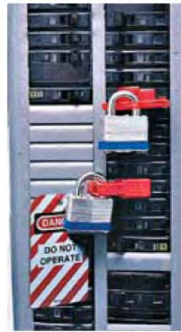
Danger tagged circuit breaker locking off devices
